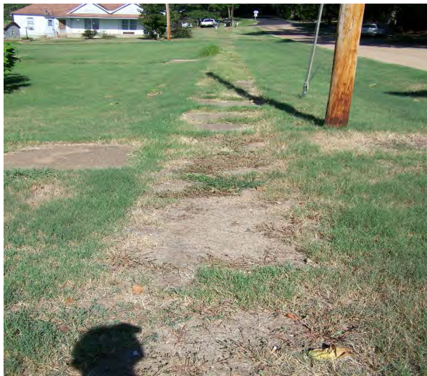
Poor Condition: Green Street facing west
