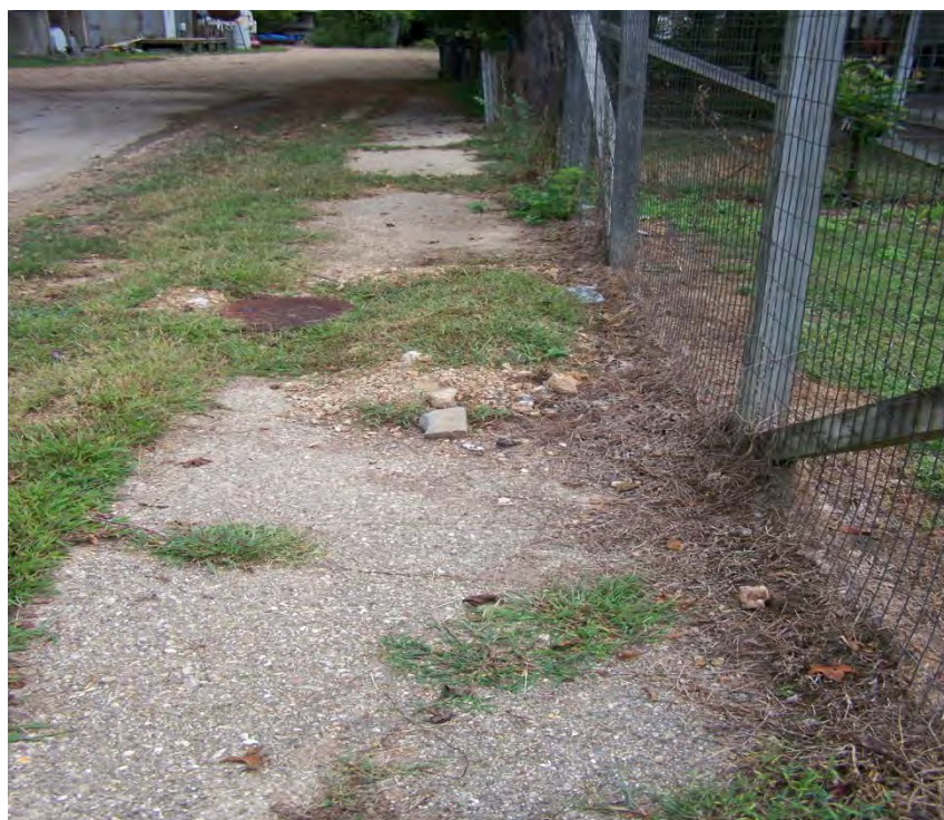
Poor Condition: Main Street North of Maple
