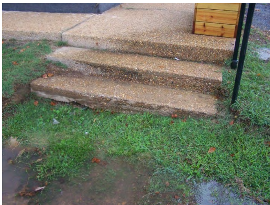
Poor Condition: Main Street facing south
