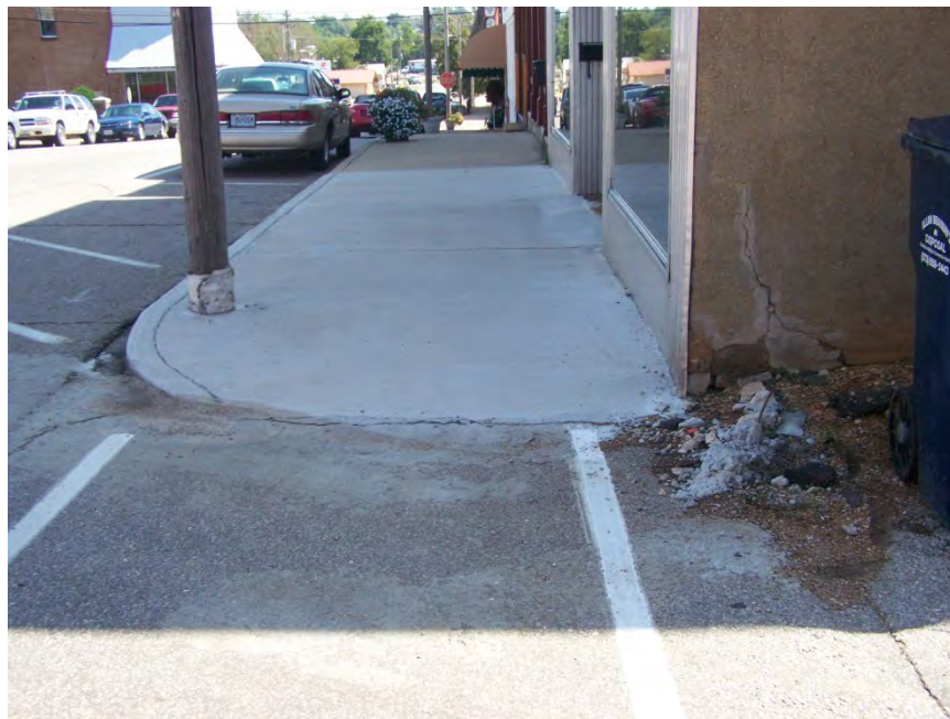
Good Condition: Washington and Charles Streets
