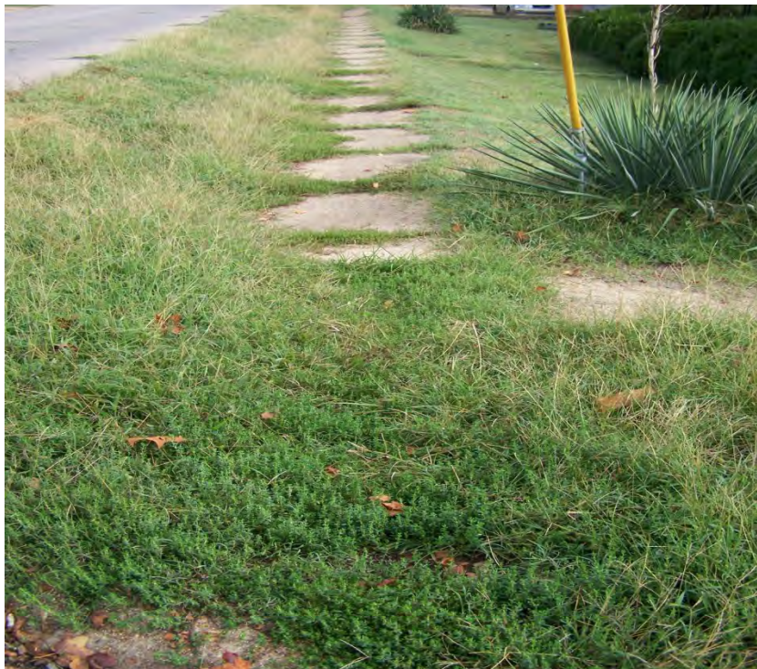
Poor Condition: Young Street west of Walnut
